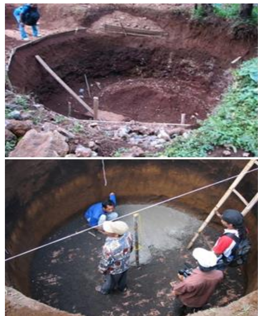
Figure 4. The process of digging the reactor pit and strengthening the foundation floor
